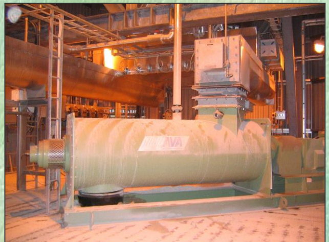
Mixer for moistening of the ash.
