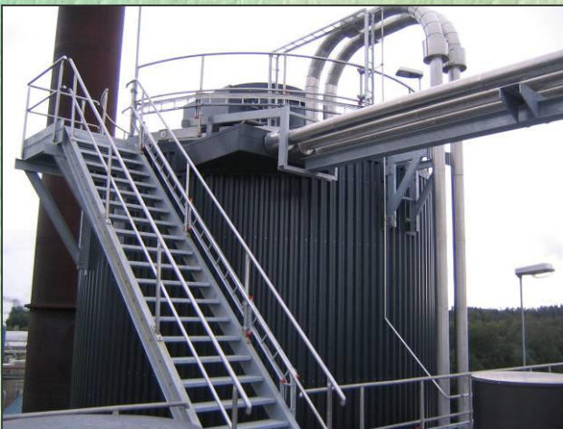
Five inlet pipes in the top of the silo.
